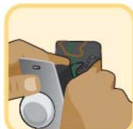
Fold the wires back into the box.
